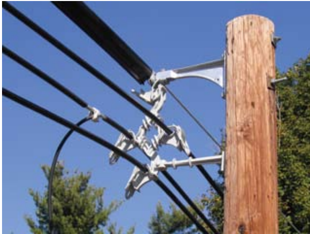
15 kV Spacer Cable System
