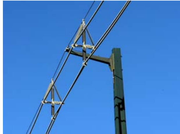
69 kV Spacer Cable System
