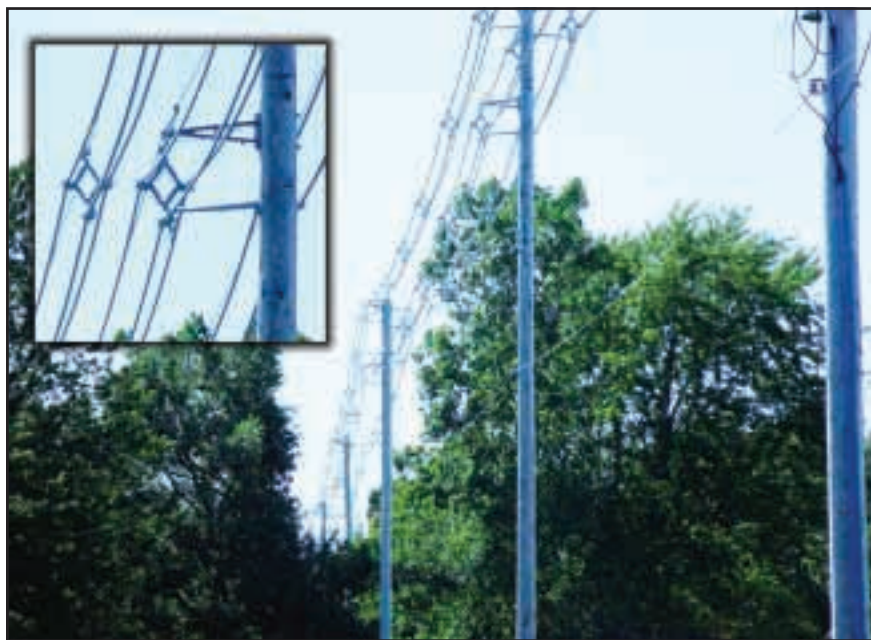
A typical example of aerial spacer cable construction involving multiple paralleled circuits.
