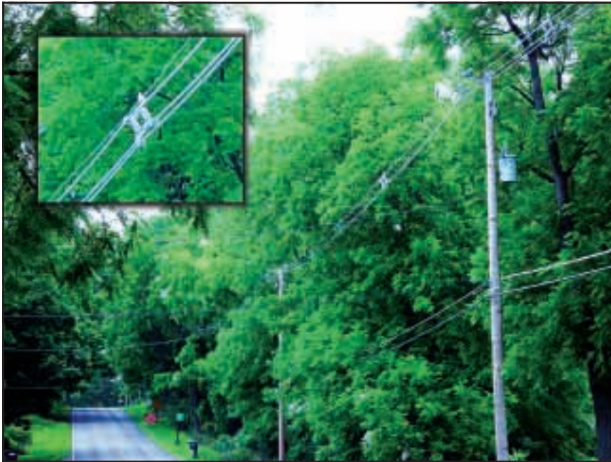
A typical aerial spacer cable system with tree-tolerance capabilities.
